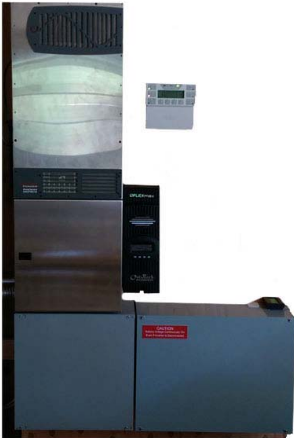
Fig 2. Radian inverter with charge controller, MATE3 monitoring display and battery storage 4kw version with 10kwh storage
